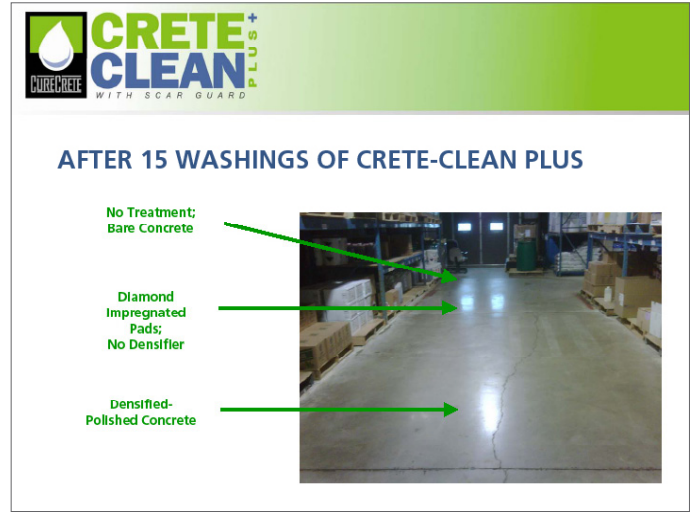
After 15 washings with CreteClean Plus with Scar Guard, the improvement in the floor's sheen is magnified even further.
